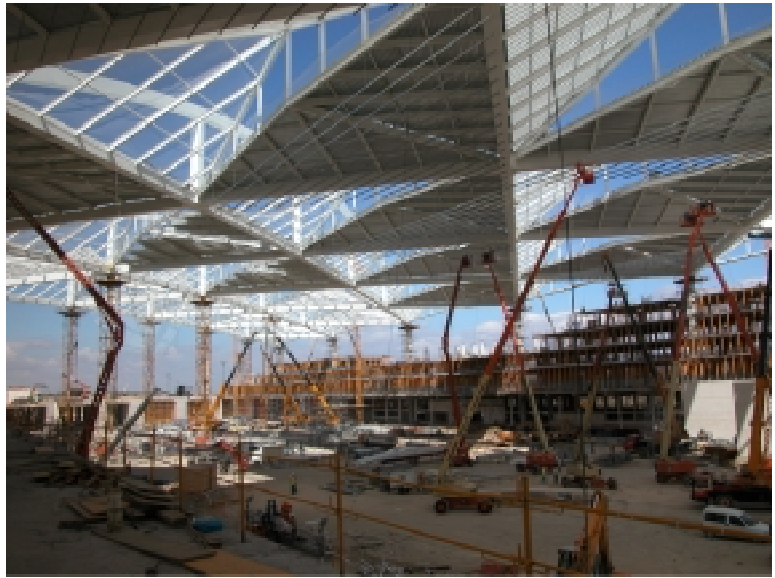
Fig. 6 Roof with changes to the original project of the secondary structure (Photo by courtesy of C. Ferrater)
