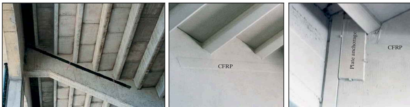
Fig. 5: Post-strengthening of existing concrete frames with externally bonded CFRP laminates: a) Before painting b) After painting c) End anchorage
